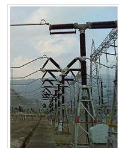
400kV SF6 circuit breakers
