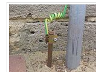
Fig. 1: A typical earthing electrode (left of gray conduit) at a home in Australia. Note the green and yellow marked earth wire.
