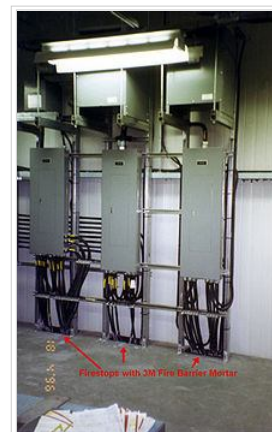
Electrical panels in an electrical service room at St. Mary's Pulp and Paper, Sault Ste. Marie, Ontario, Canada, April 1996
