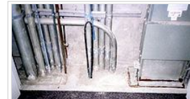
Topside of firestop with penetrants consisting of electrical conduit on the left and a bus duct on the right. The firestop consists of firestop mortar on top and rockwool on the bottom, for a 2 hour fire-resistance rating.
