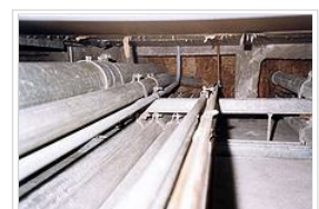
Electrical Conduit risers, seen inside fire-resistance rated shaft, as seen entering bottom of a firestop. The firestop is made of firestop mortar on top, rockwool on the bottom. Raceways are used to protect cables from damage.
