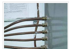
Mineral insulated cables at a panel board
