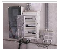
a modern "fuse box" - a distribution board using MCBs, next to a box with an embedded power meter
