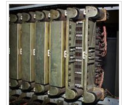
Several 30-contact relays in "Connector" circuits in mid 20th century 1XB switch and 5XB switch telephone exchanges; cover removed on one
